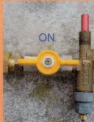
Turn yellow isolator to ON
